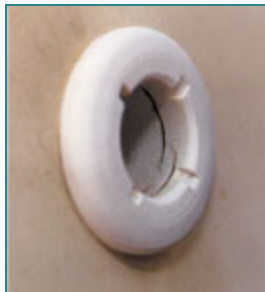
Plastic thru-hulls turn brittle and eventually crack from ultraviolet (UV) sunlight. Failures usually occur inside the thru-hull opening. If the thru-hull is only an inch or two above the waterline, rainwater or snow accumulations can force it underwater and sink the boat.
